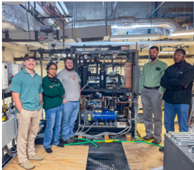
Hot Gas Bypass Chiller
