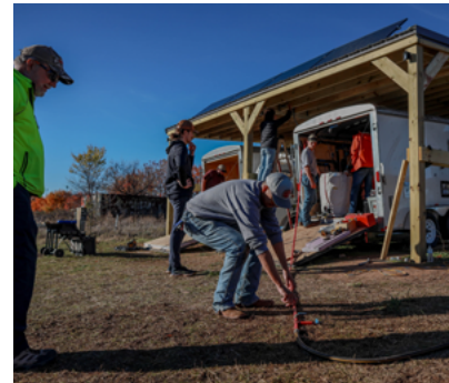
Off-Grid Heating and Cooling system for a tiny house 2024 Spring & Fall
